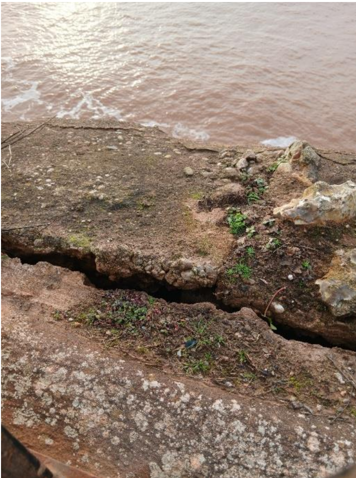
Photo of crack opened up since last inspection.
